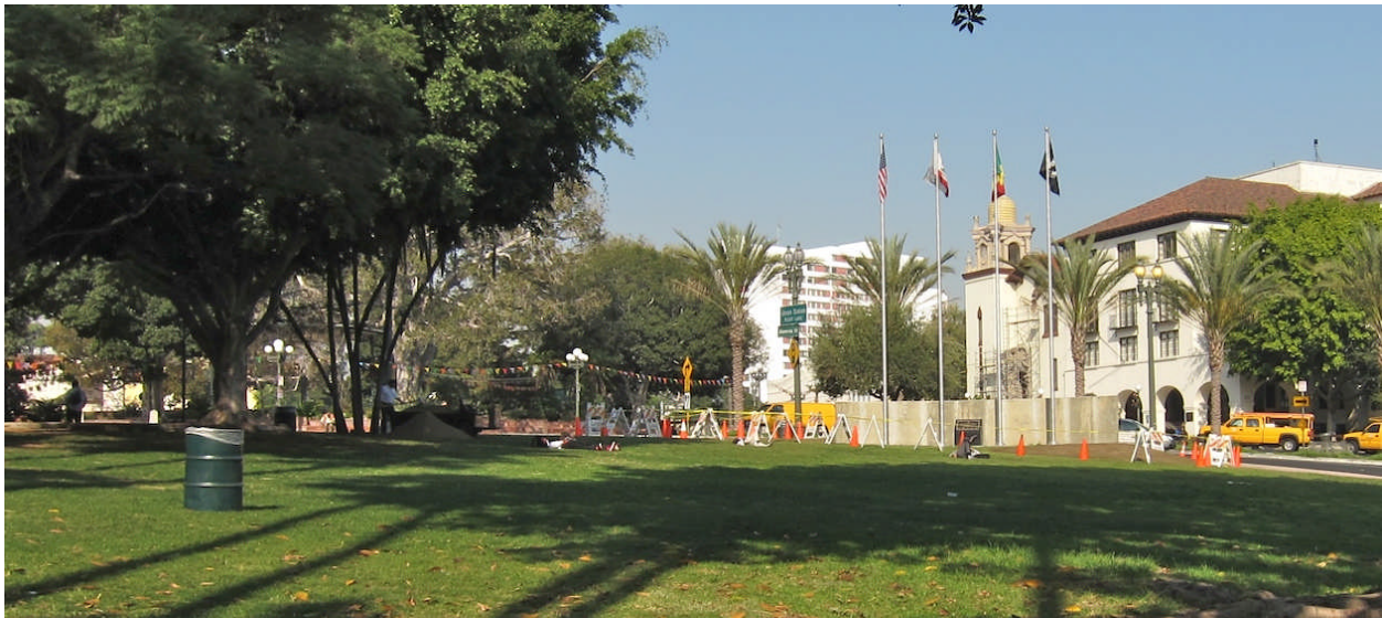
Father Serra Park in El Pueblo de Los Angeles Historic Monument showing the Project wall under construction on November 19, 2009.
